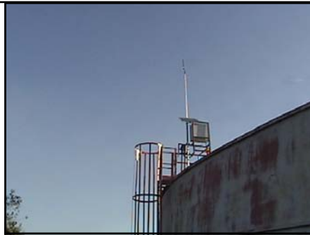
Wireless I/O, solar panel, and antenna mounted on water tank
