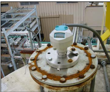
Radar level transmitter mounted on nozzle
