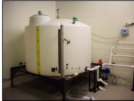
Gilson Engineering indoor flow and level lab
