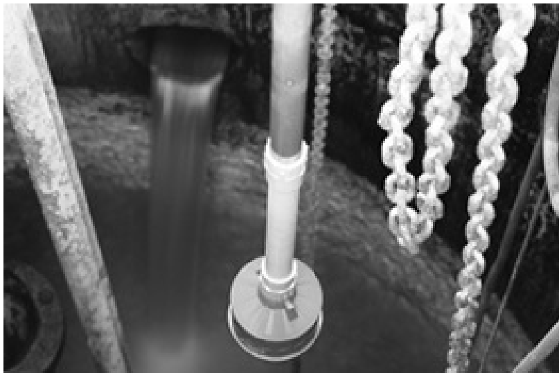
Monitoring level in sewage wet well
