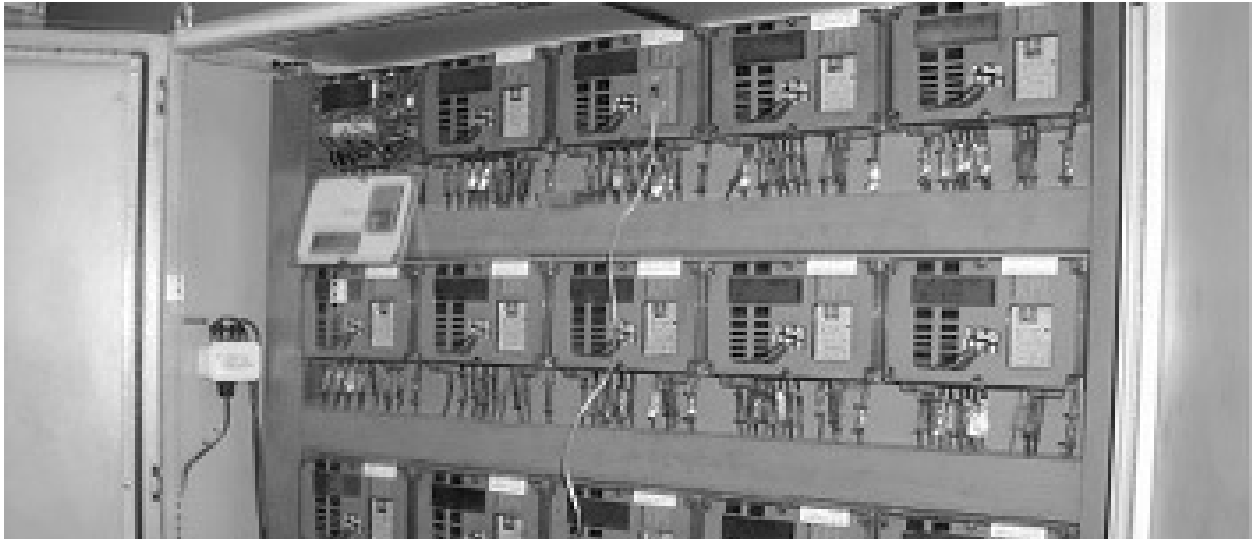
SITRANS LU10 monitoring coal bunkers
