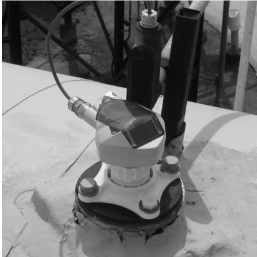
Sulfuric acid storage
