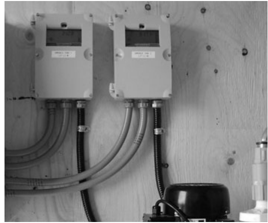
Two MultiRangers measuring ammonia tanks
